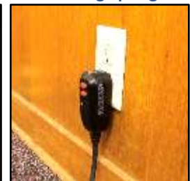
Ground Fault Protected
