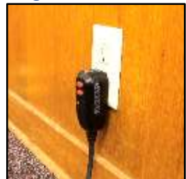
Ground Fault Protected
